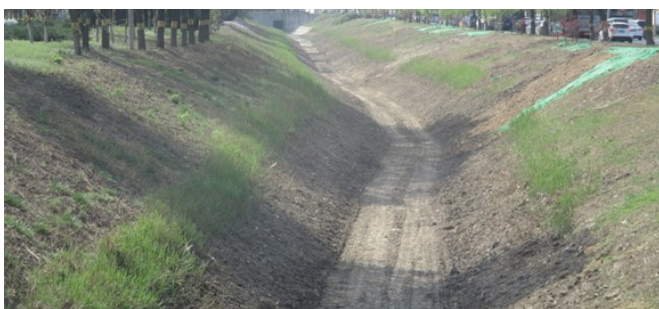
Figure 4b Comparison Before and After Renovation of A Section of A Small and Medium-Sized River in Beijing
